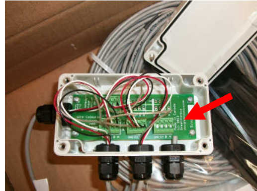
Figure 5 Open Auxiliary Box
